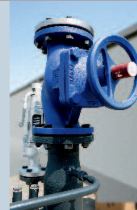
Steam outlet and safety valve
